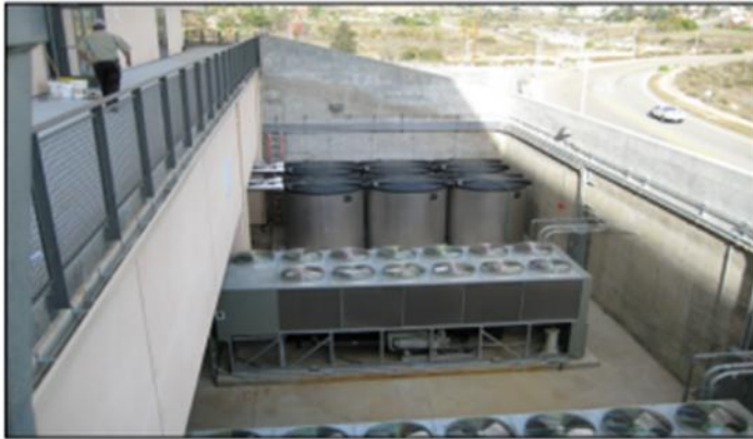
5 MW Thermal Storage – LA Community College (Calmac)
