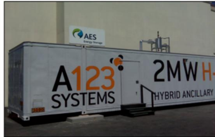
2 MW Li-Ion Battery for A/S – AES (A123)
