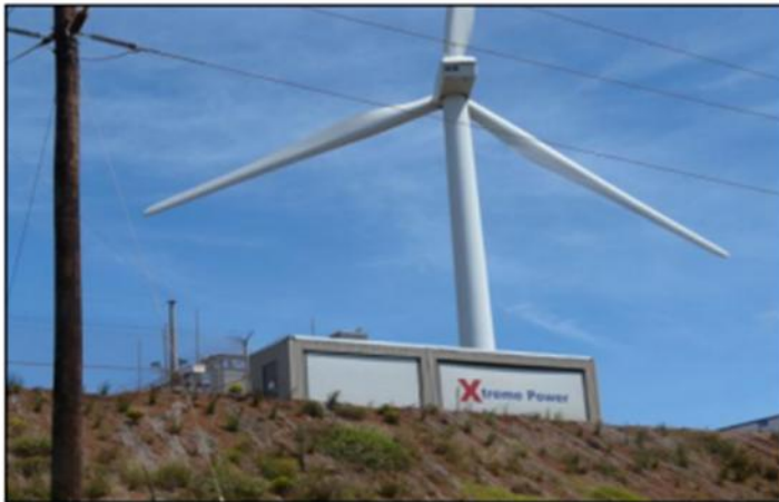
1 MWh Battery in Maui, Hi (Xtreme Power)
